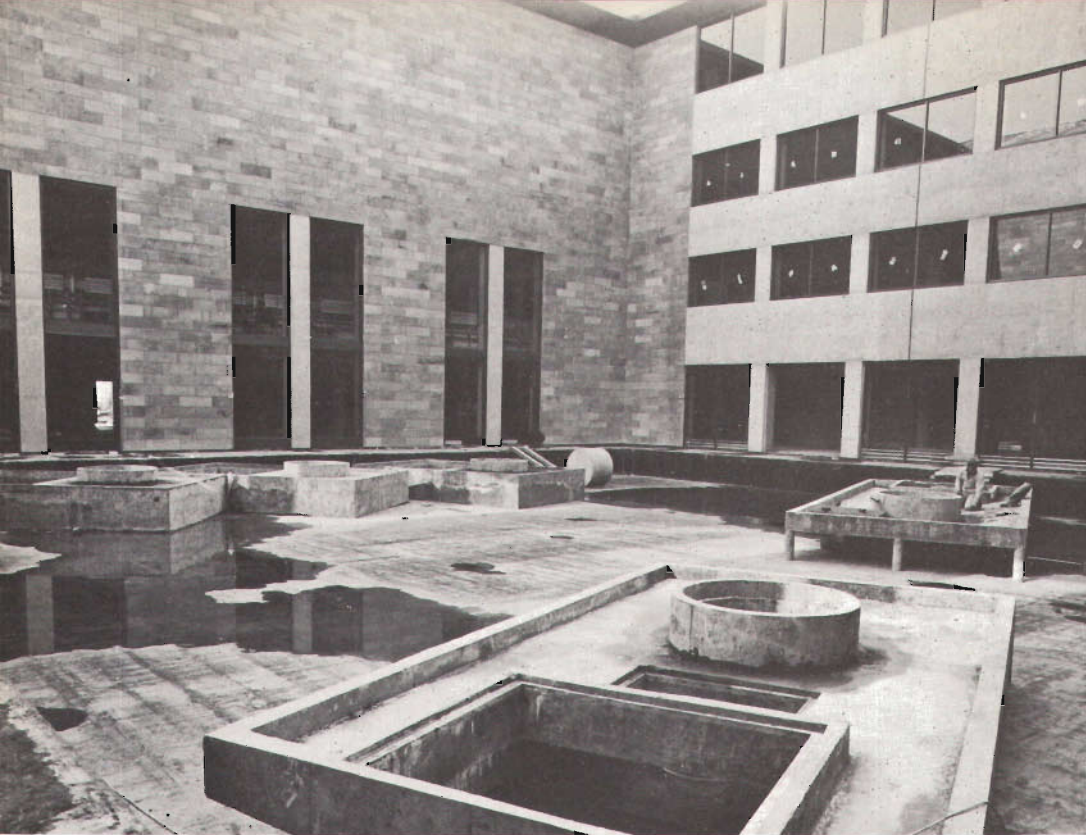
Basic structure of the flooring and hydraulic installations in the Oriental Courtyard. [National Gallery of Victoria
